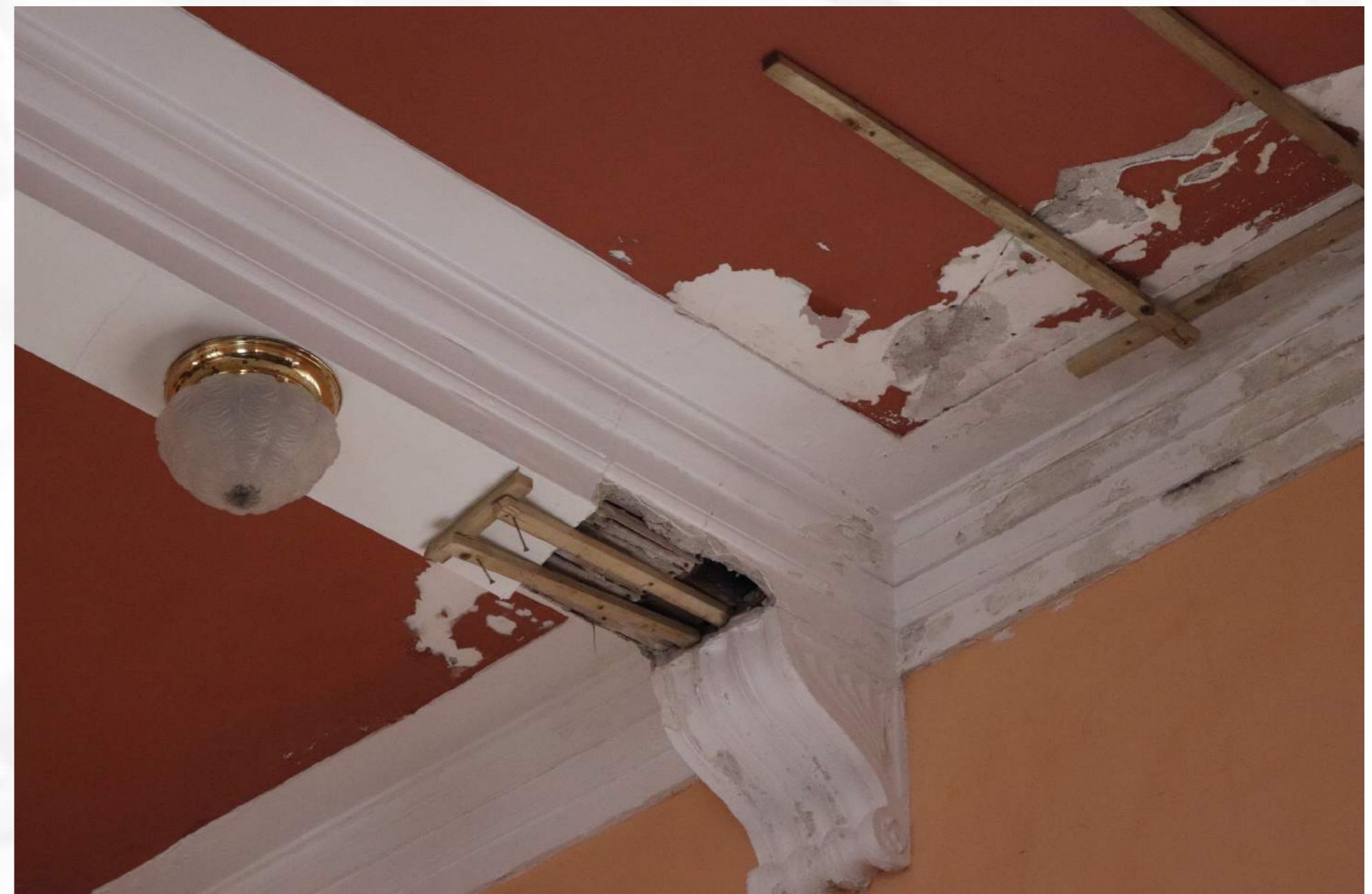
Symptoms of Damp Ingress Within The Guildhall The root cause relates to poor roof detailing
