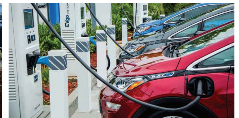
Electric vehicle charging points
