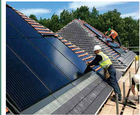
Integrated Solar Panels
